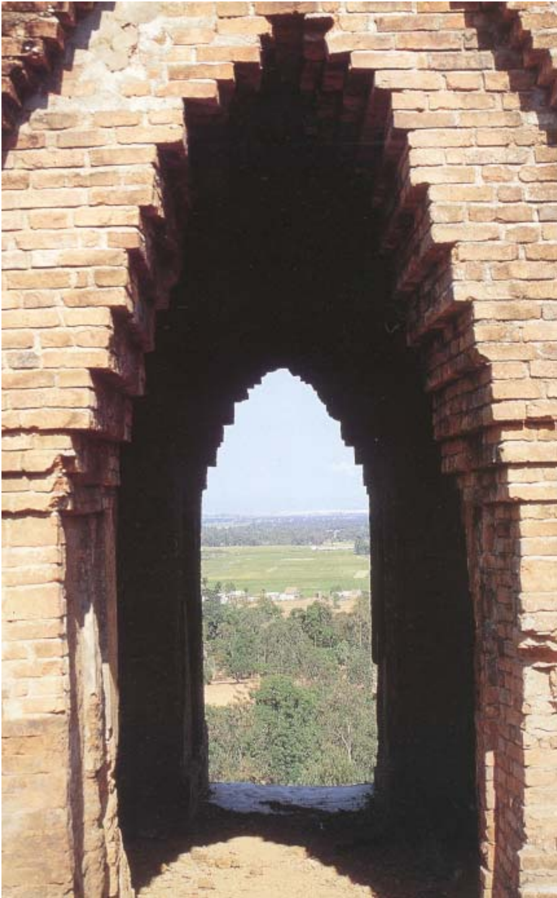
View of a Cham tower. 12th century C.E. Brick with sandstone elements, Thoc Loc, north of Quy Nhon, by Bin Dinh, South Vietnam.
